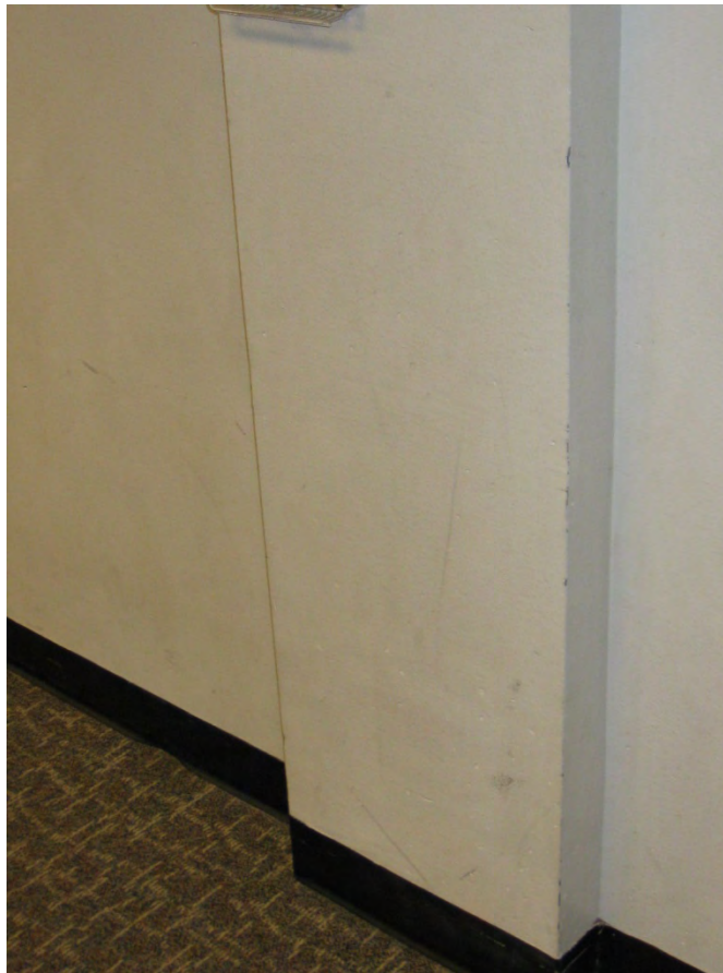
Typical condition of interior gypsum wallboard at multipurpose rooms
