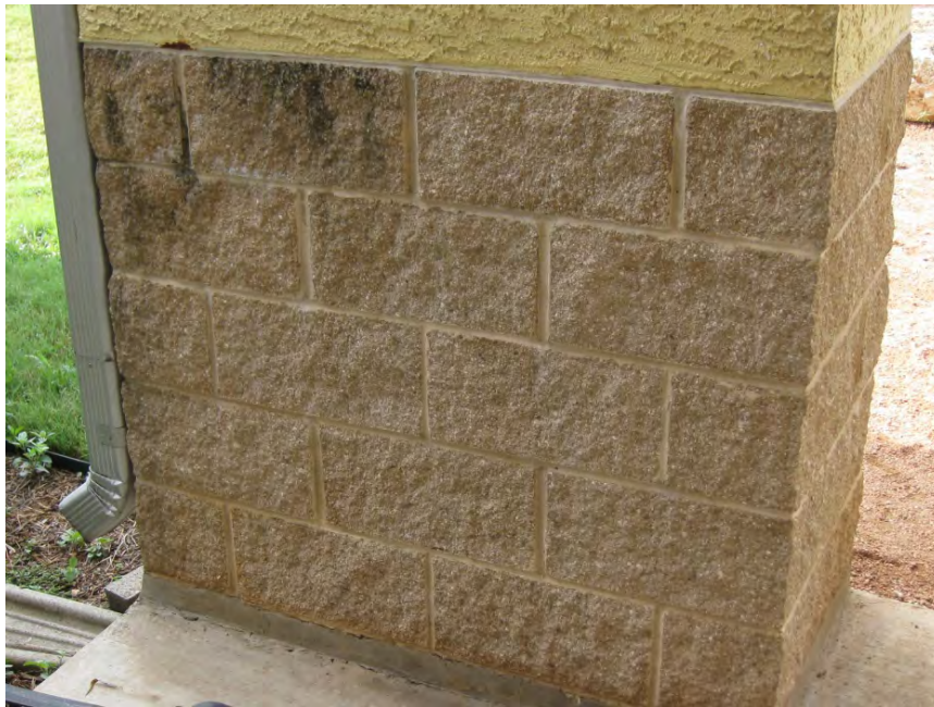
Evidence of surface mold at the entry columns
