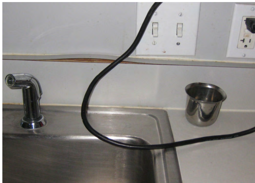
Image showing delamination of plastic laminate counters in kitchen
