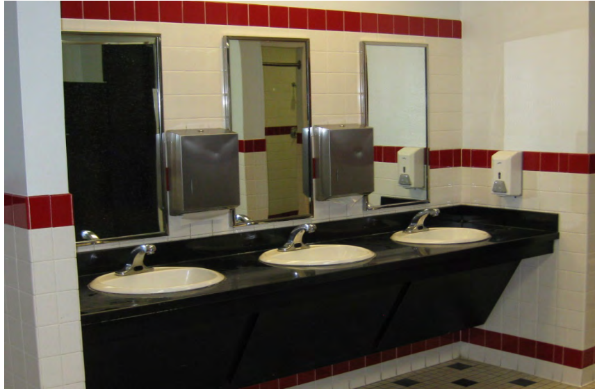
Image showing good condition of the solid surface countertops at public toilets
