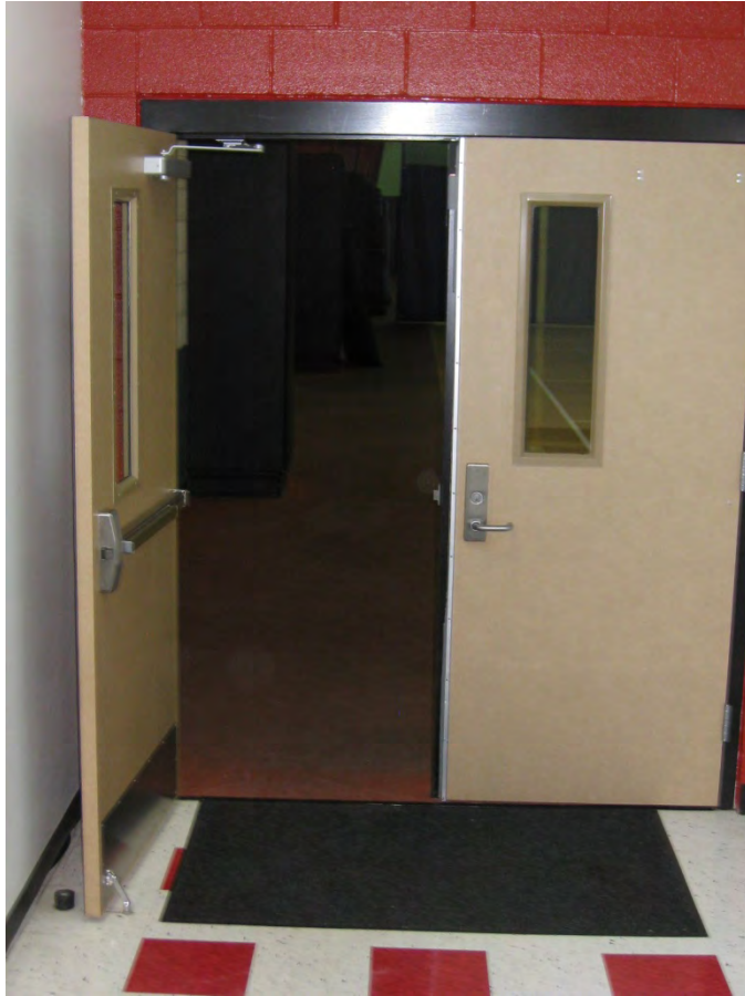
Interior door at gym is typical of the good condition of all interior doors
