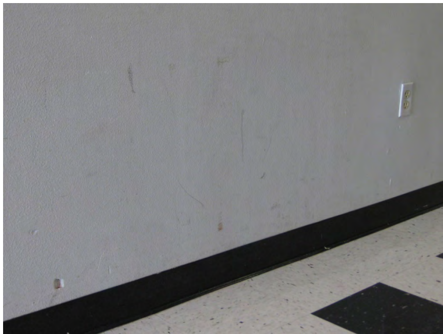
Interior gypsum wallboard damage in east corridor
