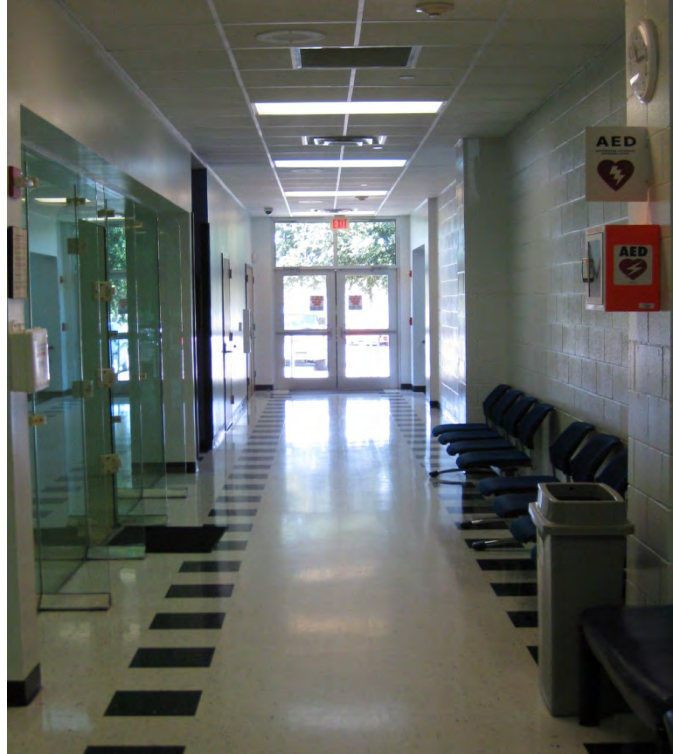
Image of overall condition of west corridor floors
