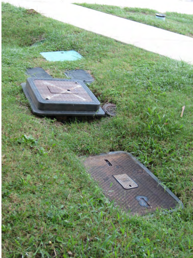
Image of in ground utilities at the west side of the building
