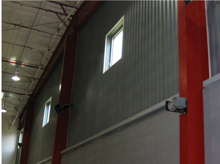
Interior painted concrete masonry units (CMU) and metal wall panels at gym
