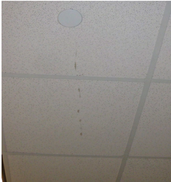
Typical level of ceiling damage at multipurpose rooms
