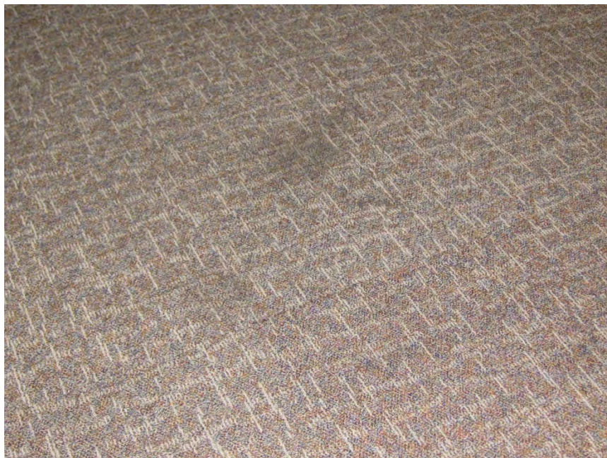
Sample of stained carpet tiles in multipurpose rooms
