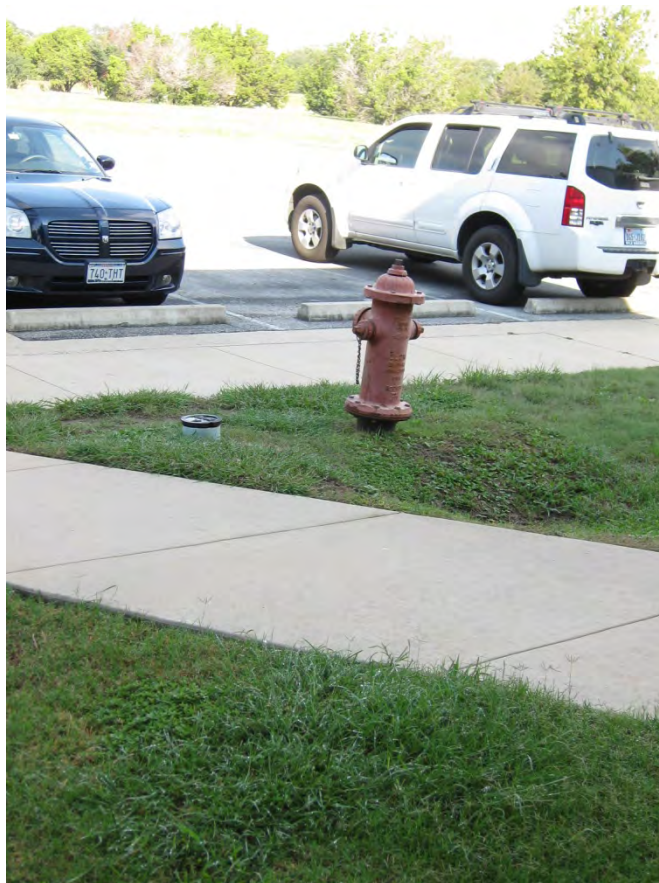
Image of fire hydrant at west side of the building
