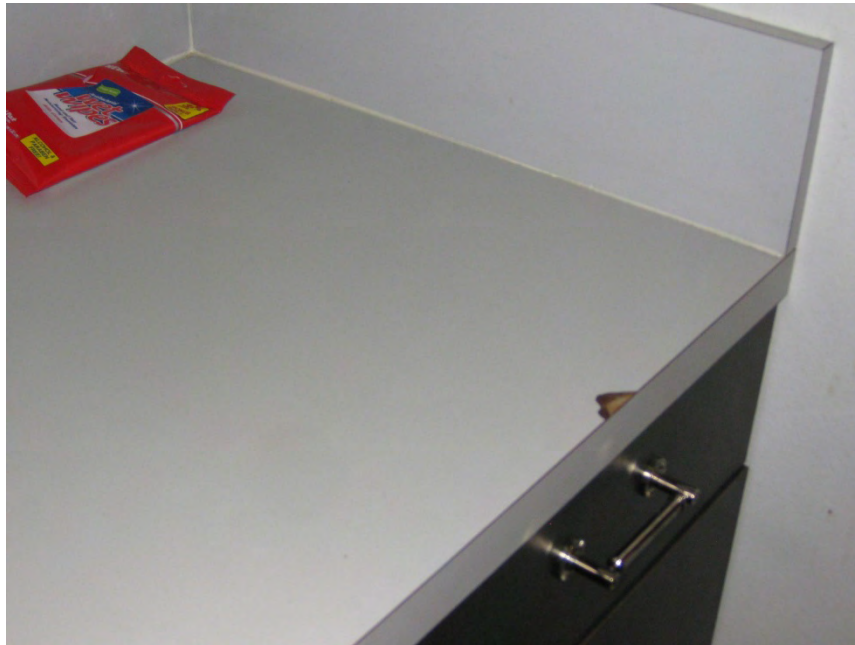
Image showing wear and tear of the plastic laminate counters in the kitchen
