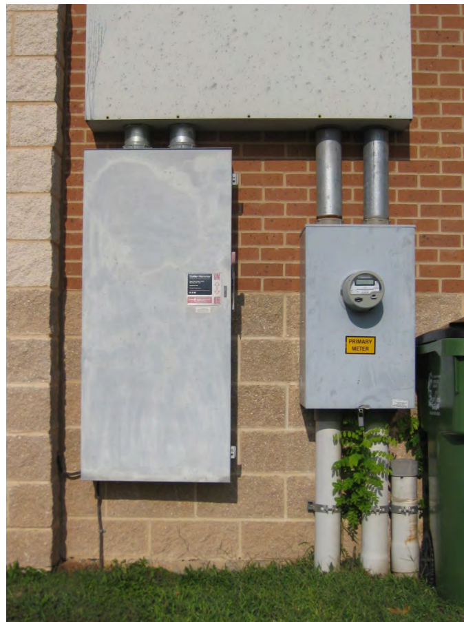
Electrical Service Entry at east side of building
