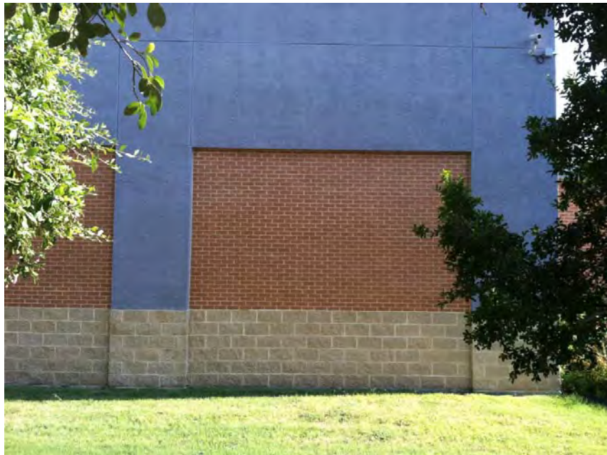
Example of Concrete Masonry Units (CMU), brick, plaster and metal wall panels
