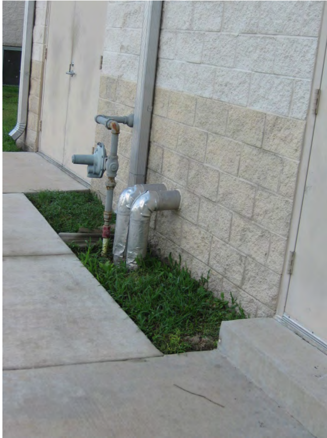
Image of gas regulator at west side of the building
