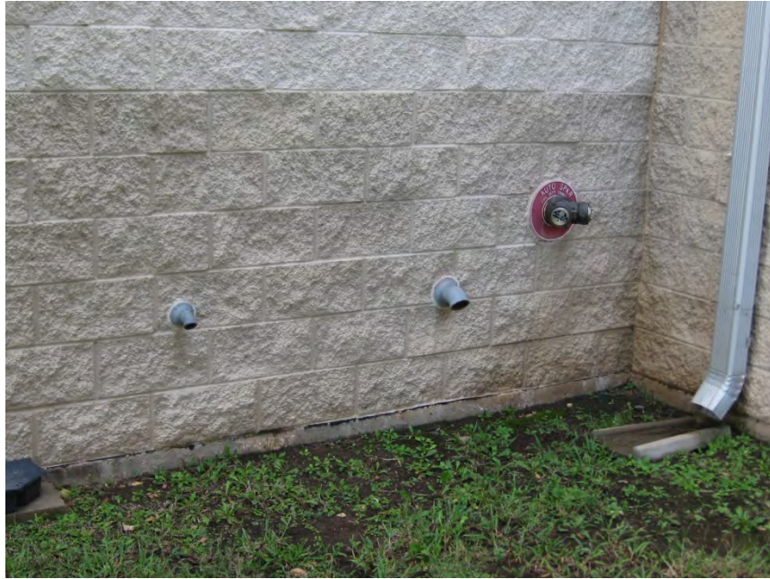
Image of fire department connection at fire riser room
