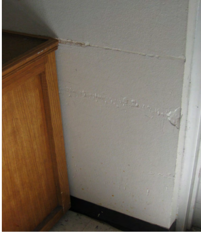
Interior gypsum wallboard damage in east corridor
